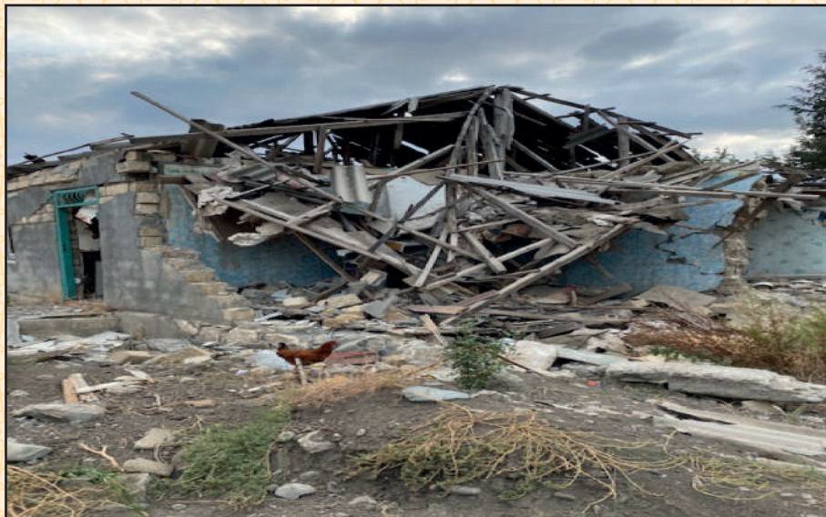
Damaged House in Terter Cityt
